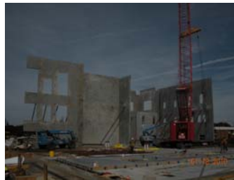
Building 3, Tilt-Panel Erection St. Cloud High School James A. Cummings, Inc. BRPH Architects/Engineers
